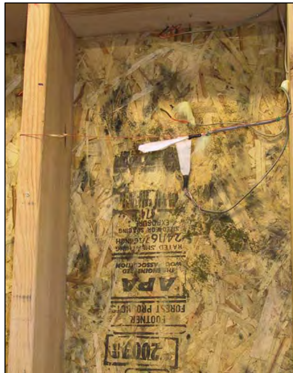
Figure 5. Mold resulting from inadequate vapor retarder control on Wall 7
